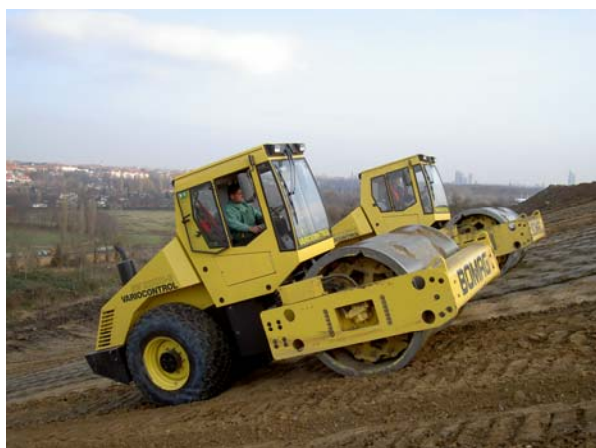
Fig. 13: Two single drum rollers with polygonal drum during compaction of the equalising layer
