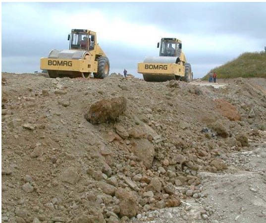
Fig. 11: Compaction of filled layers ranging from 1 m to 1.5 m at Hahn airport
